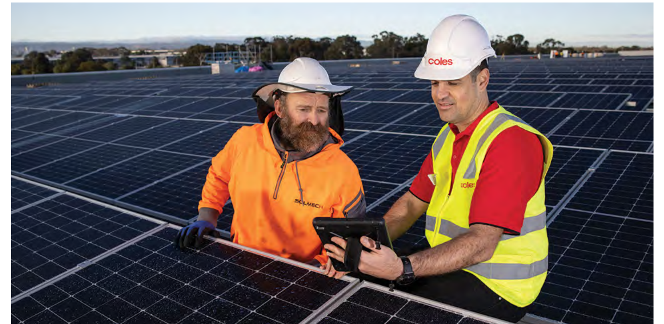
Solar installer Garry and Coles team member Michael review the installation of panels at Coles' distribution centre at Edinburgh Parks in South Australia.
